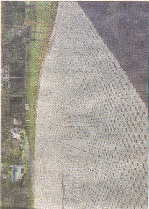
Porous pavers being used in a parking lot: In some situations, materials like these can reduce the amount of runoff that flows into rivers and streams.
