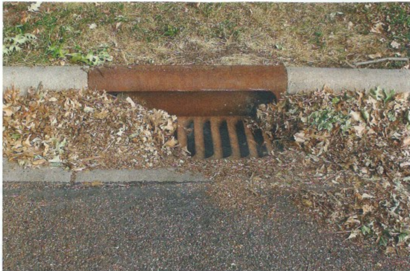
Figure 1. Storm grate with leaf accumulation
